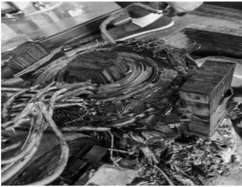
图6 一次绕组烧毁情况 Fig. 6 Burning condition of primary winding
